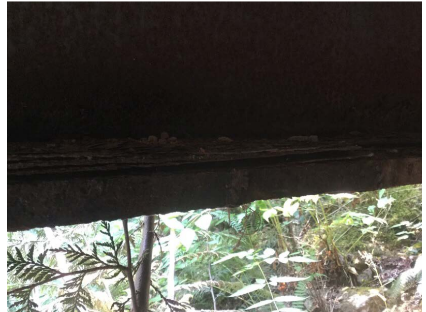
Minor steel delamination on bottom flanges
