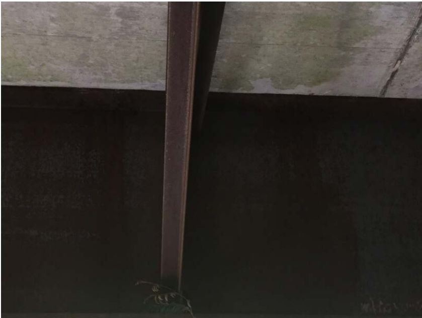
Water getting through some grout pockets - 5% of pockets
