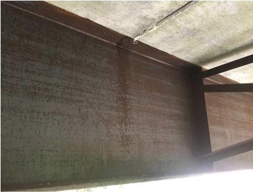
Water getting through some deck joints - 50% of joints but only minor corrosion
